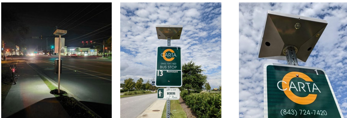
Solar lights and shelter lights installed at CARTA stops.
