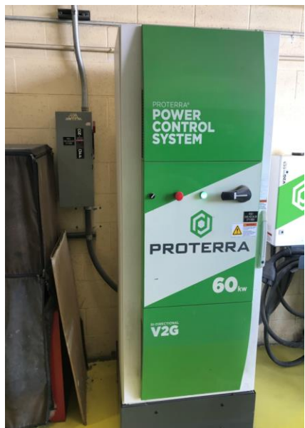
Figure 34: Charging cabinet and dispenser within maintenance bay
