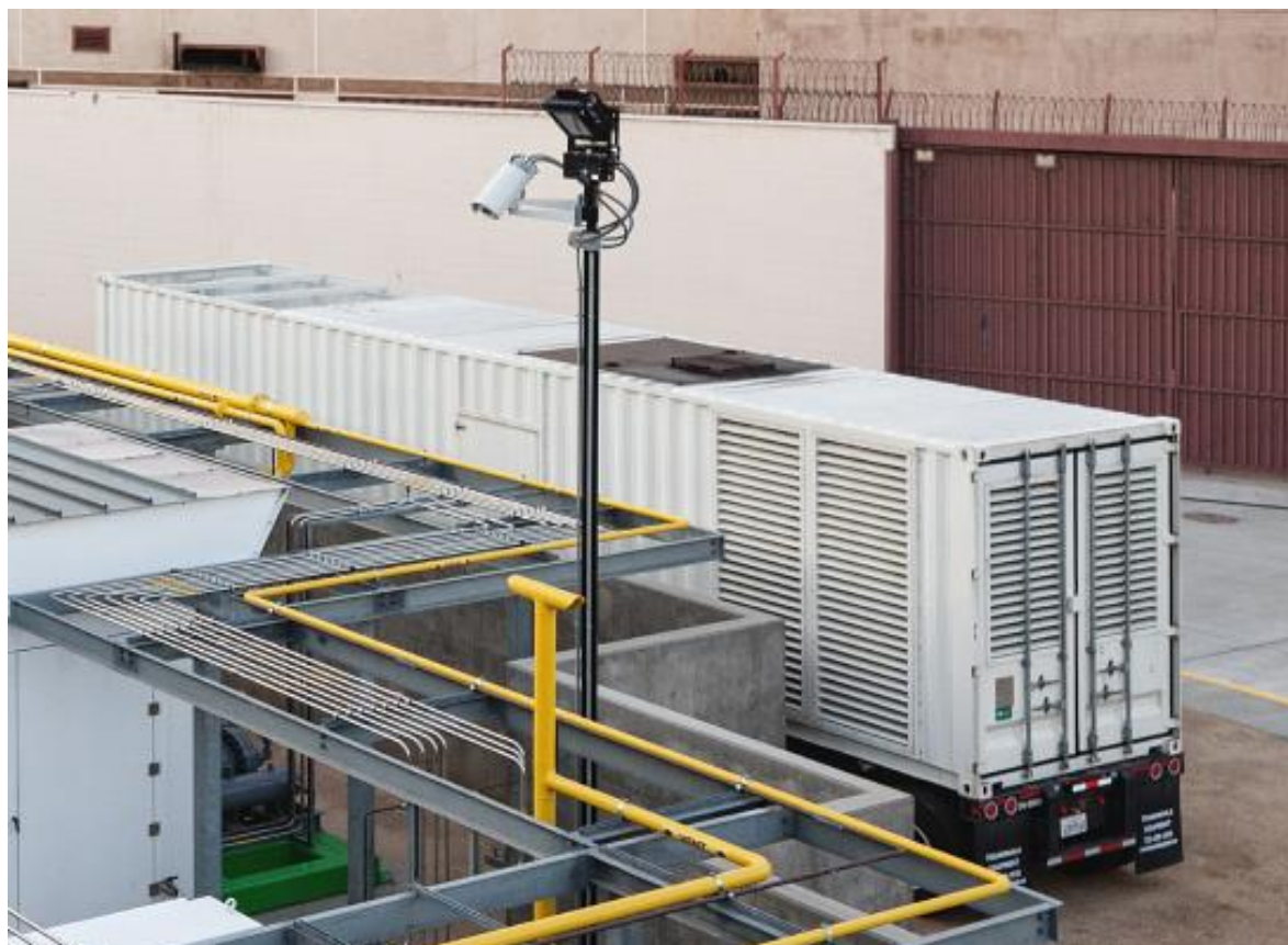
Figure 35: Backup mobile diesel generator at LA Metro Division 13, Los Angeles, CA.
