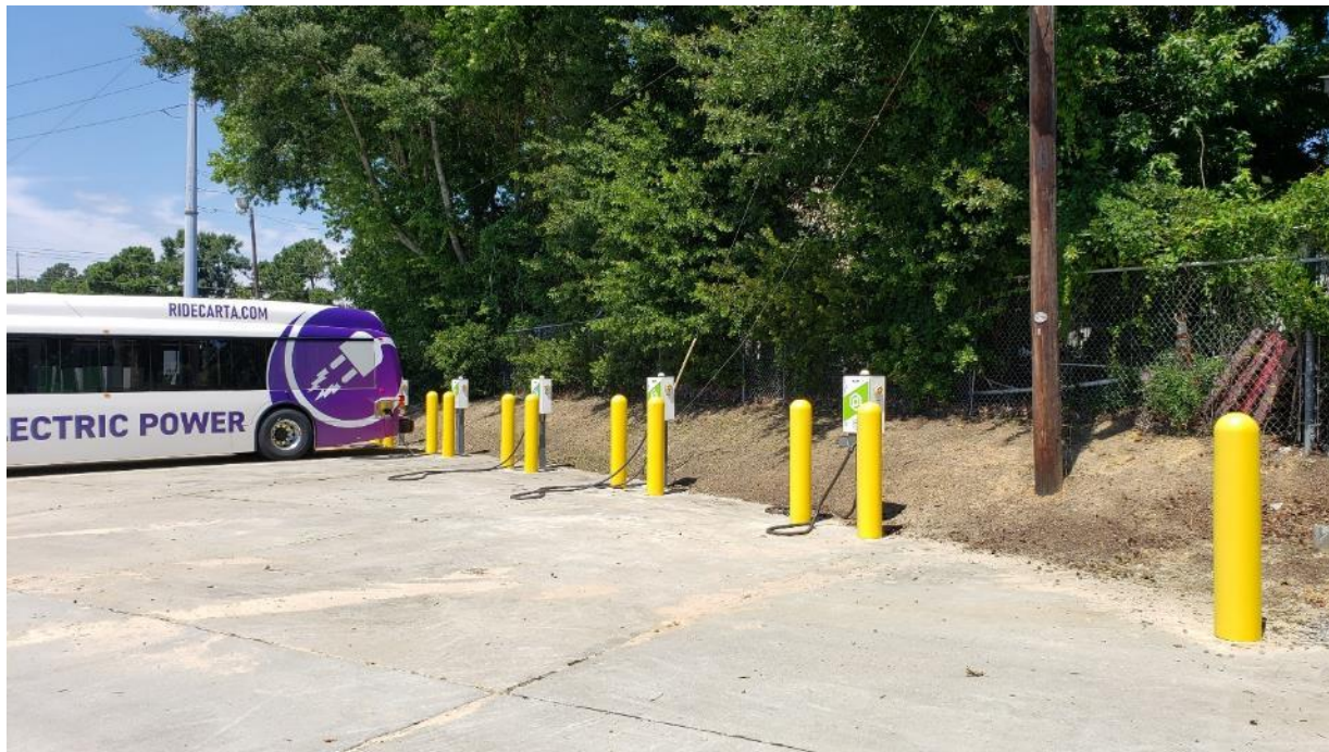
Figure 40: Electrical charging dispensers (five of six total dispensers visible)
