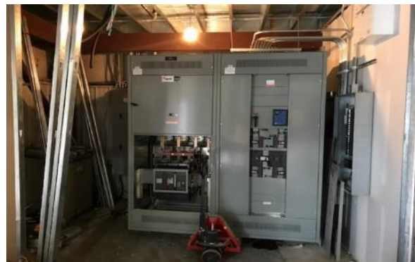
New/ Modified Switchgear
