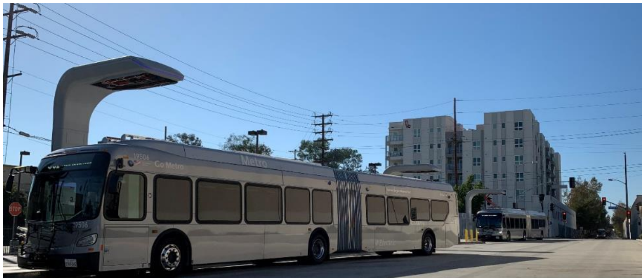
Figure 10: LA Metro’s on-route/layover charging at the North Hollywood bus-rail station.
