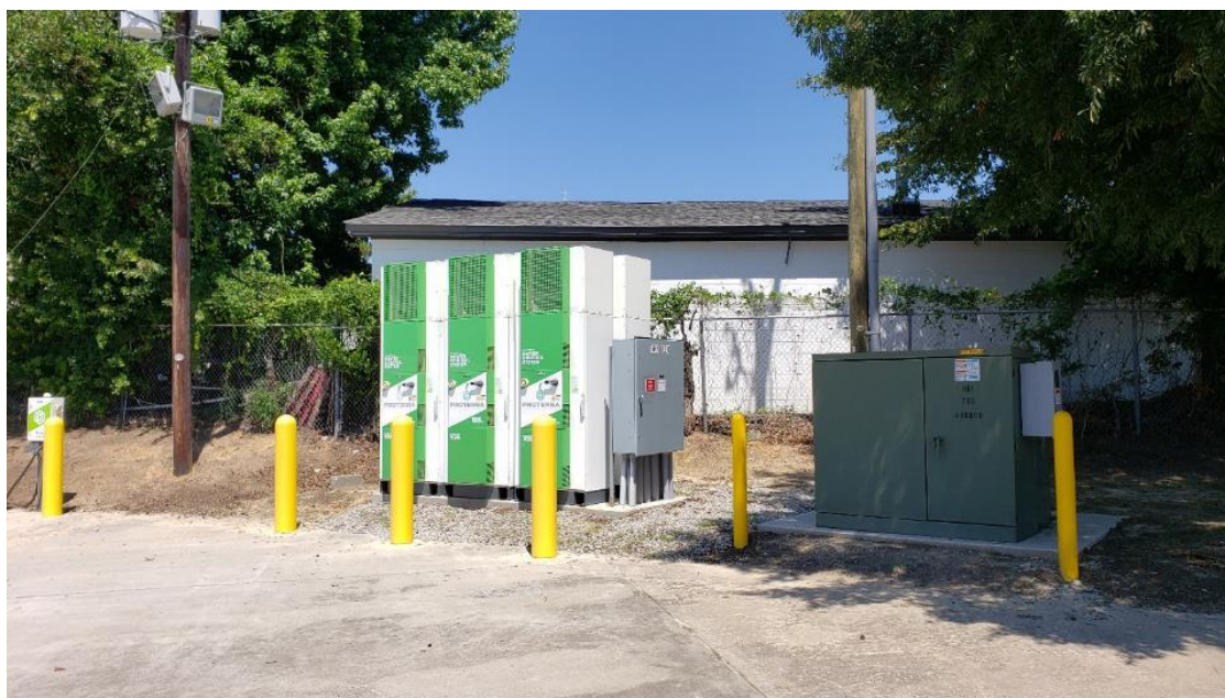
Figure 41: Electrical charging station array (six units - 125 kW per unit)
