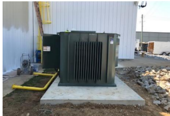
Upgraded Service Transformer
