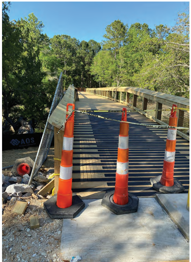
The new bicycle/pedestrian bridge will provide a safe connection between neighborhoods on either side of Jeremy Creek
